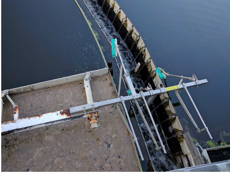
Weir Brush System – Clarifier 4
