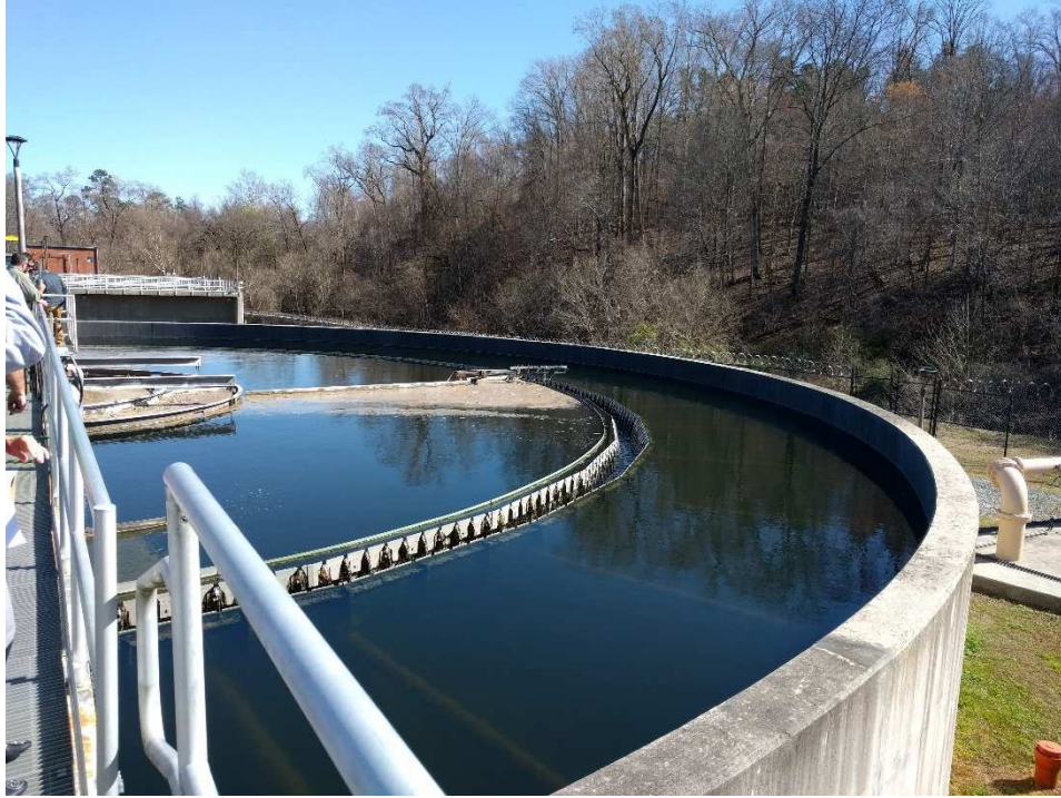
Inboard Effluent Launder – Clarifier 4
