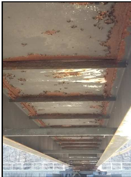
Photo 10: Severe rust is seen on the underside of the checker plate
