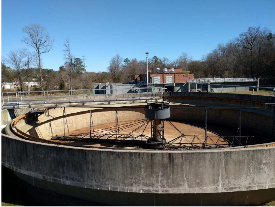
Undersized Centerwell with No Scum Ports - Clarifiers 2&3
