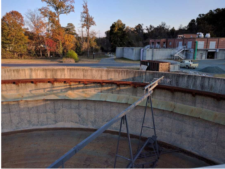
Worn Stamford Baffles – Clarifiers 2&3
