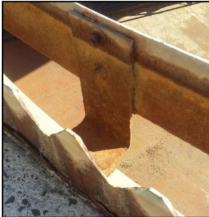
Photo 9: The current metal weirs and baffles are in a state of disrepair and need to be replacement.
