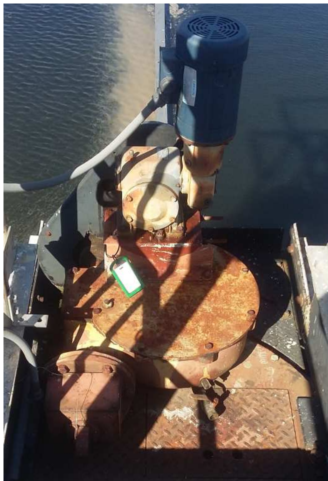
Photo 6: The drives for both clarifiers are in poor shape after operating for almost double their design life.
