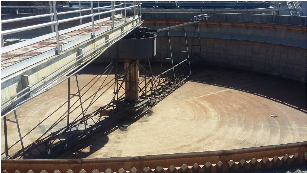
Photo 4: Envirex clarifier out of operation. Grooves are visible on the floor from the plow blades
