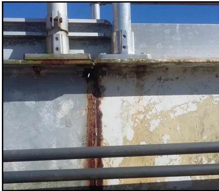
Photo 8: During the installation of the Algae Sweep/ Weir-Wolf Brush systems by Ford Hall Company, an additional section of beam bridge was added to the existing Envirex equipment.
