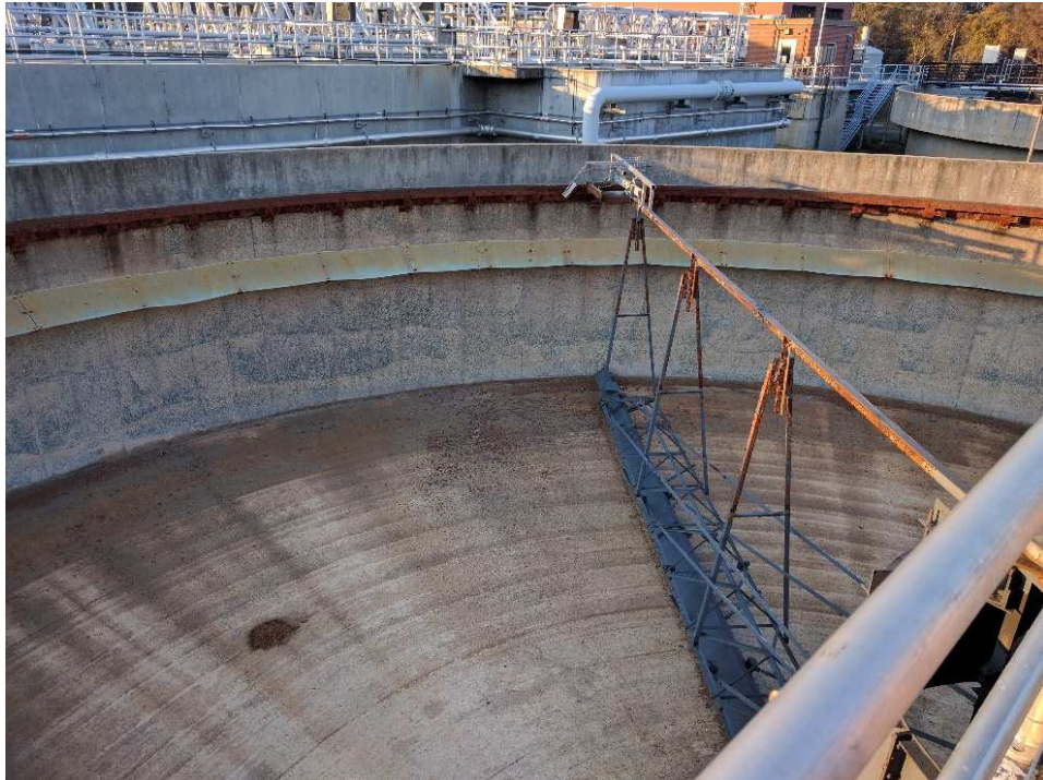
Divots in Concrete due to Unstable Centerwell – Clarifiers 2&3
