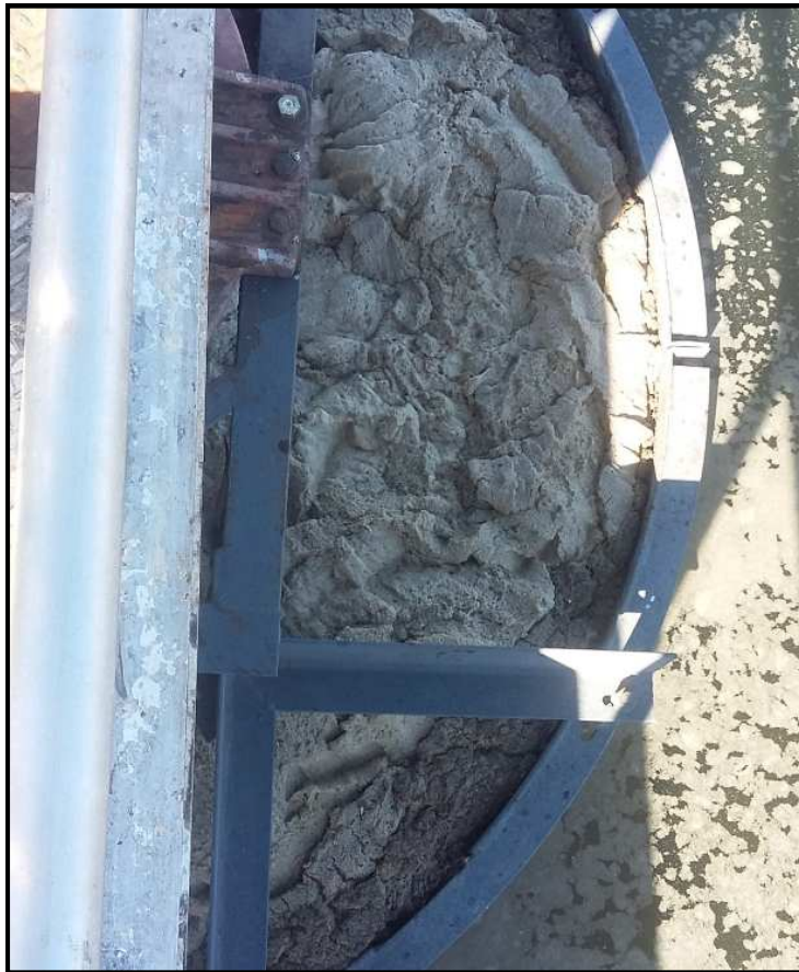
Photo 7: The existing influent well has a diameter of 8'-5". This is approximately \frac{1}{2} the size recommended for use. The purposed equipment would have an influent well of 19'-9" along with the Envirex patent FEDWA EDI.
