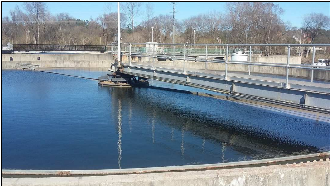
Photo 2: Envirex clarifier in operation
