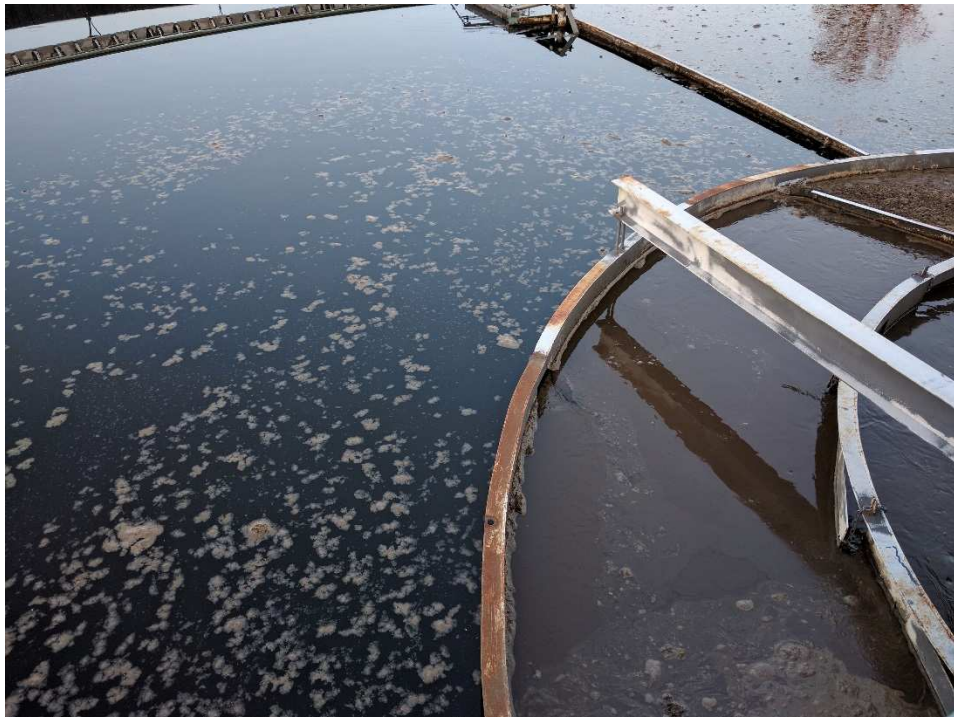
Scum Accumulation – Clarifier 4
