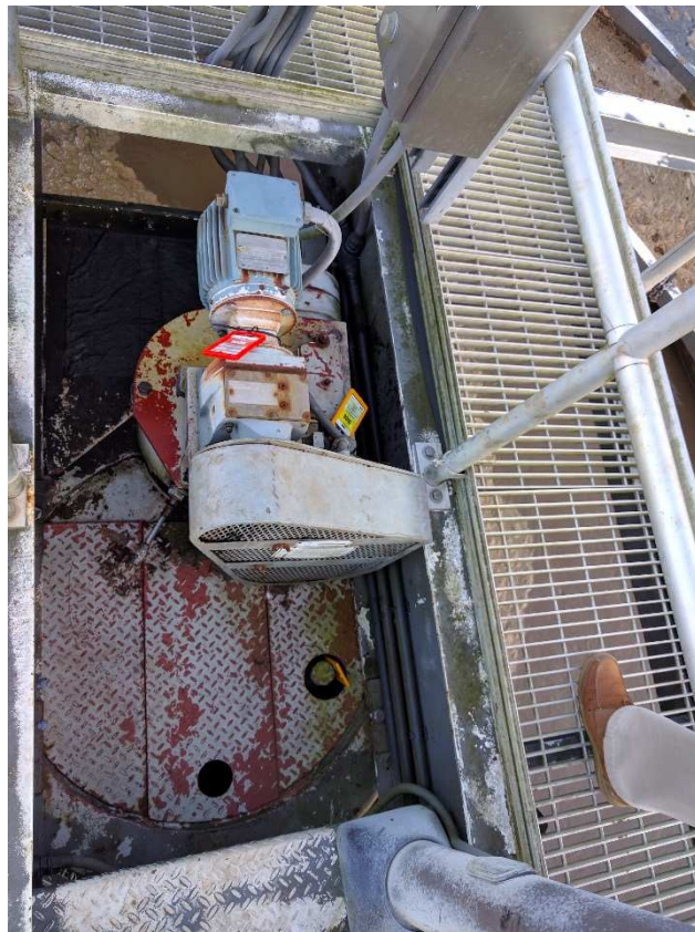
Clarifier Mechanism – Clarifier 4
