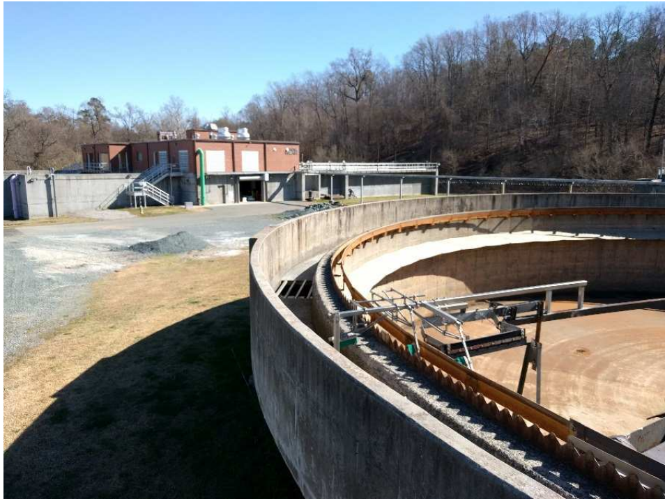
Corroded Weir Plates – Clarifiers 2&3
