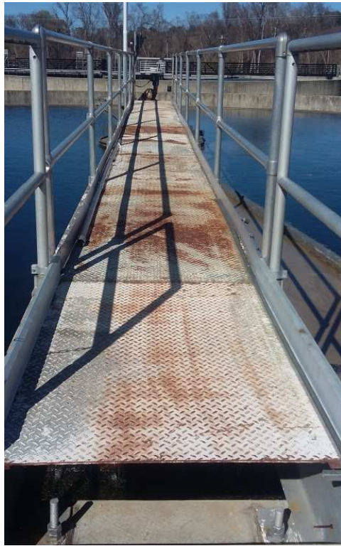
Photo 3: The above photo shows the poor condition of the existing checker plate
