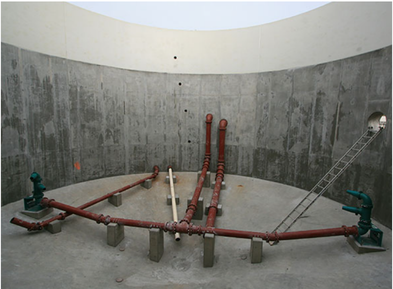
Figure 12. Example Installation of Pumped-Nozzle Mixing
