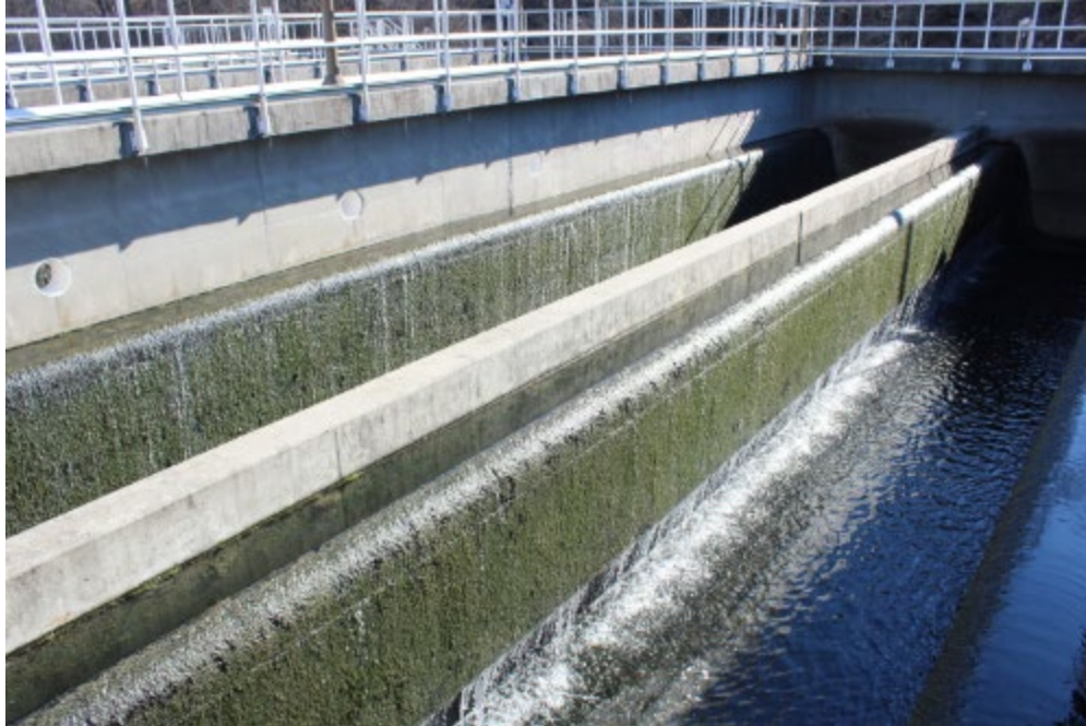
Mason Farm Wastewater Treatment Plant – Filtration System
