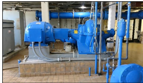
Existing Backwash Pump
