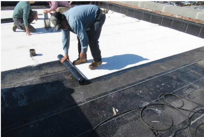
Roof replacements completed through the CIP program are prioritized through comprehensive condition assessments as part of the overall asset management program.
