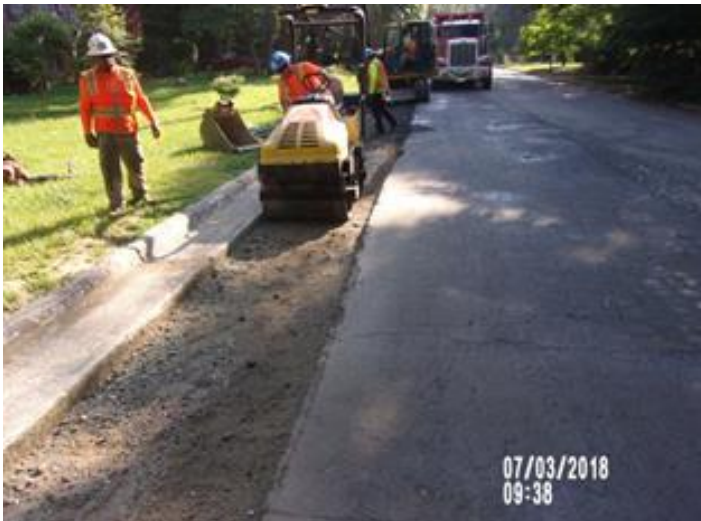
Water main replacement along Brandywine Road was completed concurrently with sewer rehabilitation throughout the Heritage Hills neighborhood.
