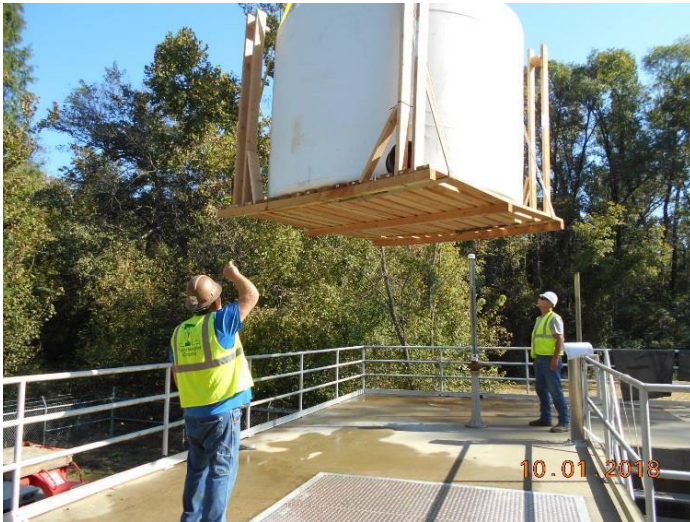
Odor control improvements are part of the second phase of $3.1 million improvements to the Rogerson Drive Pump Station
