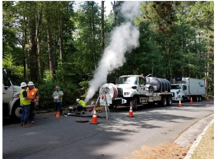
Rehabilitation using Cured-In-Place Pipe (CIPP) liner has been used to extend the life of more than 2.3 miles of sewer mains during the first half of FY 2019.
